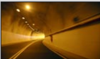
Lighting of tunnels
